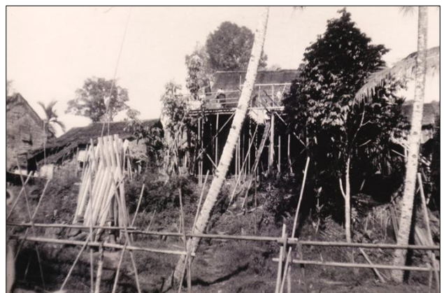
An 11 Platoon work party in Kampung Gumbang, preparing timber for use in construction.
